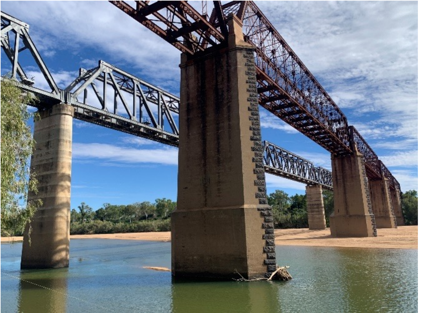
Image: Macrossan Rail Bridge over Burdekin River. Source: Charters Towers Regional Council.
